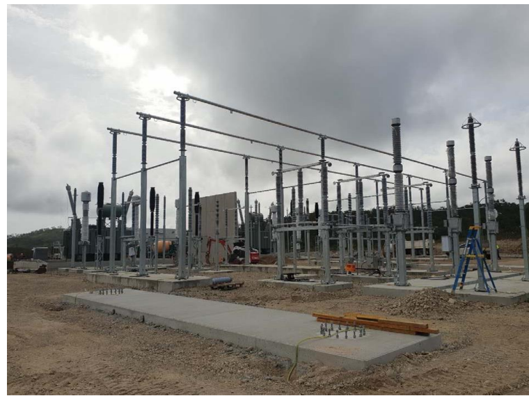
Wind farm substation powerline landing structures
