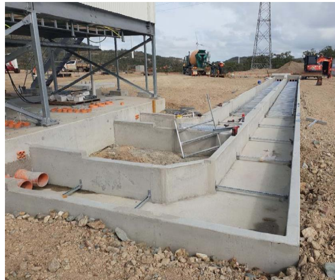
Wind farm substation cabling trenches
