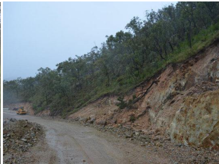
Minor bank slip on WTG11 access road
