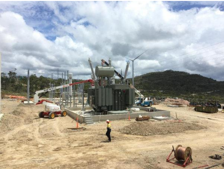
Wind farm substation
