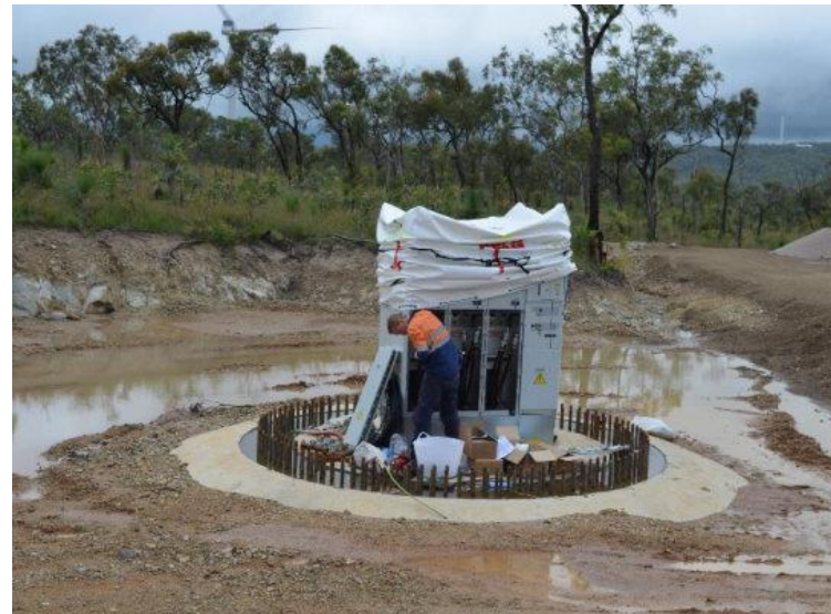
Cable termination at WTG41
