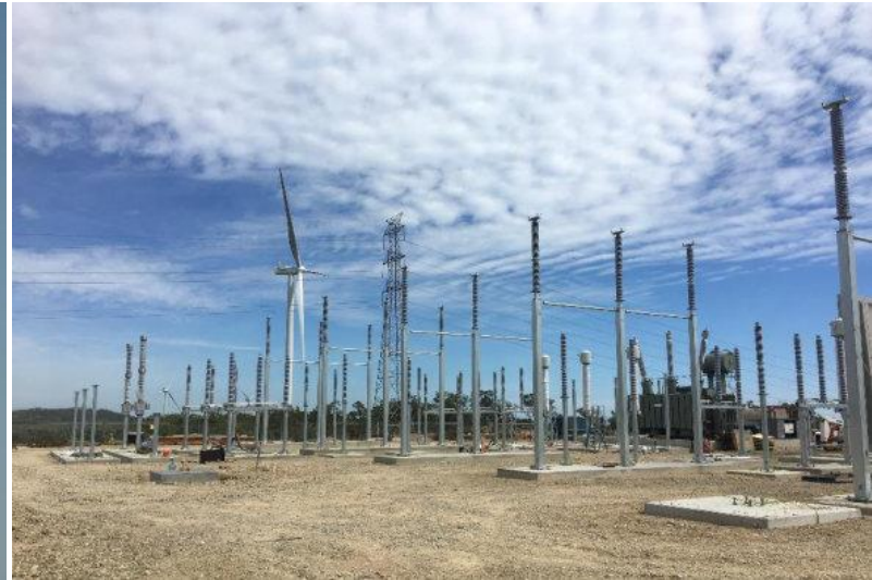
Overhead structures in Powerlink switchyard
