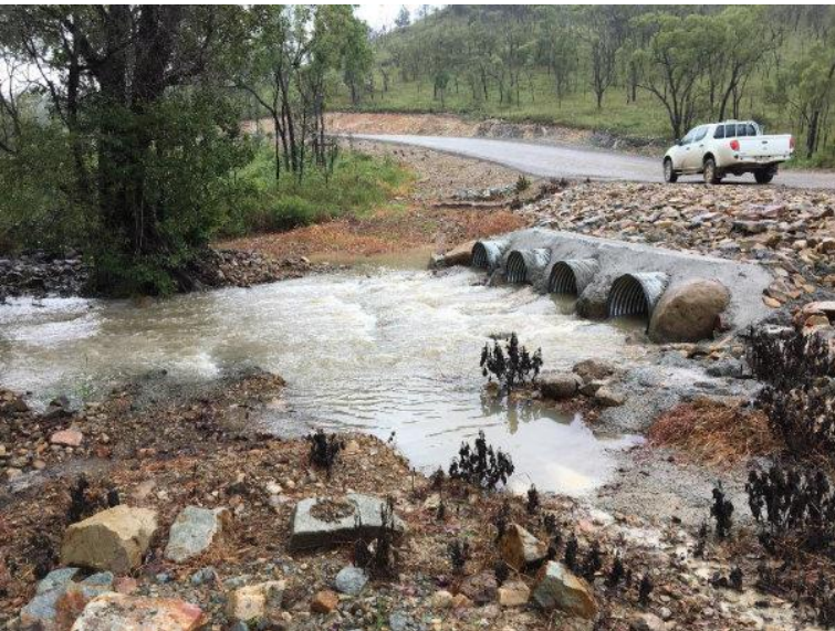
Kippen Drive culvert in action
