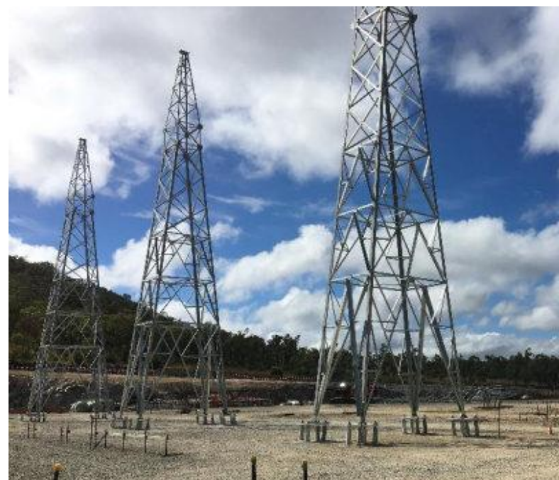
Powerlink switchyard connection towers
