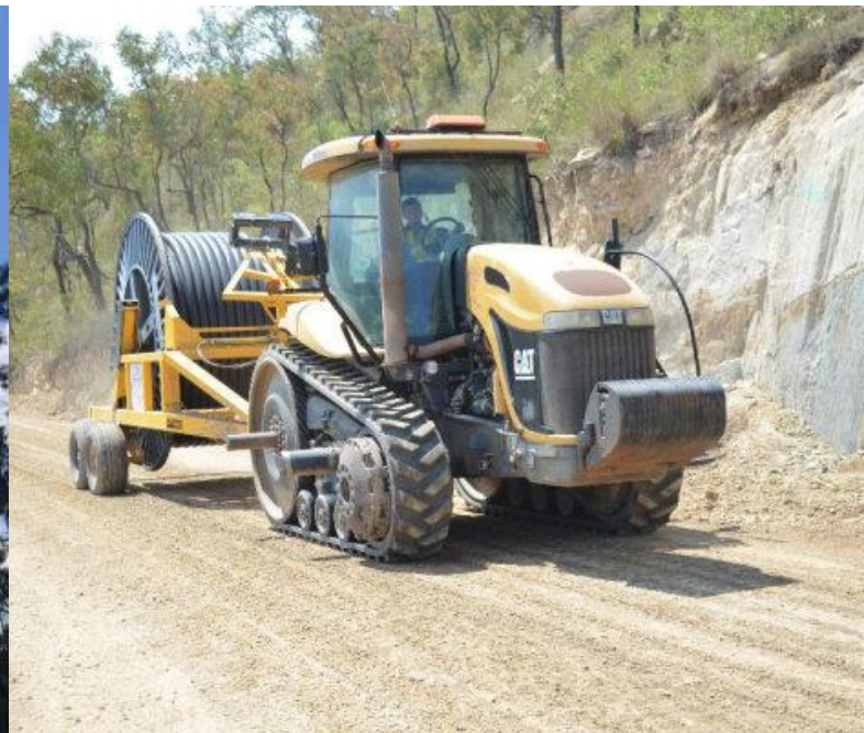
Underground cable transport
