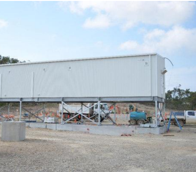
Substation Control Building
